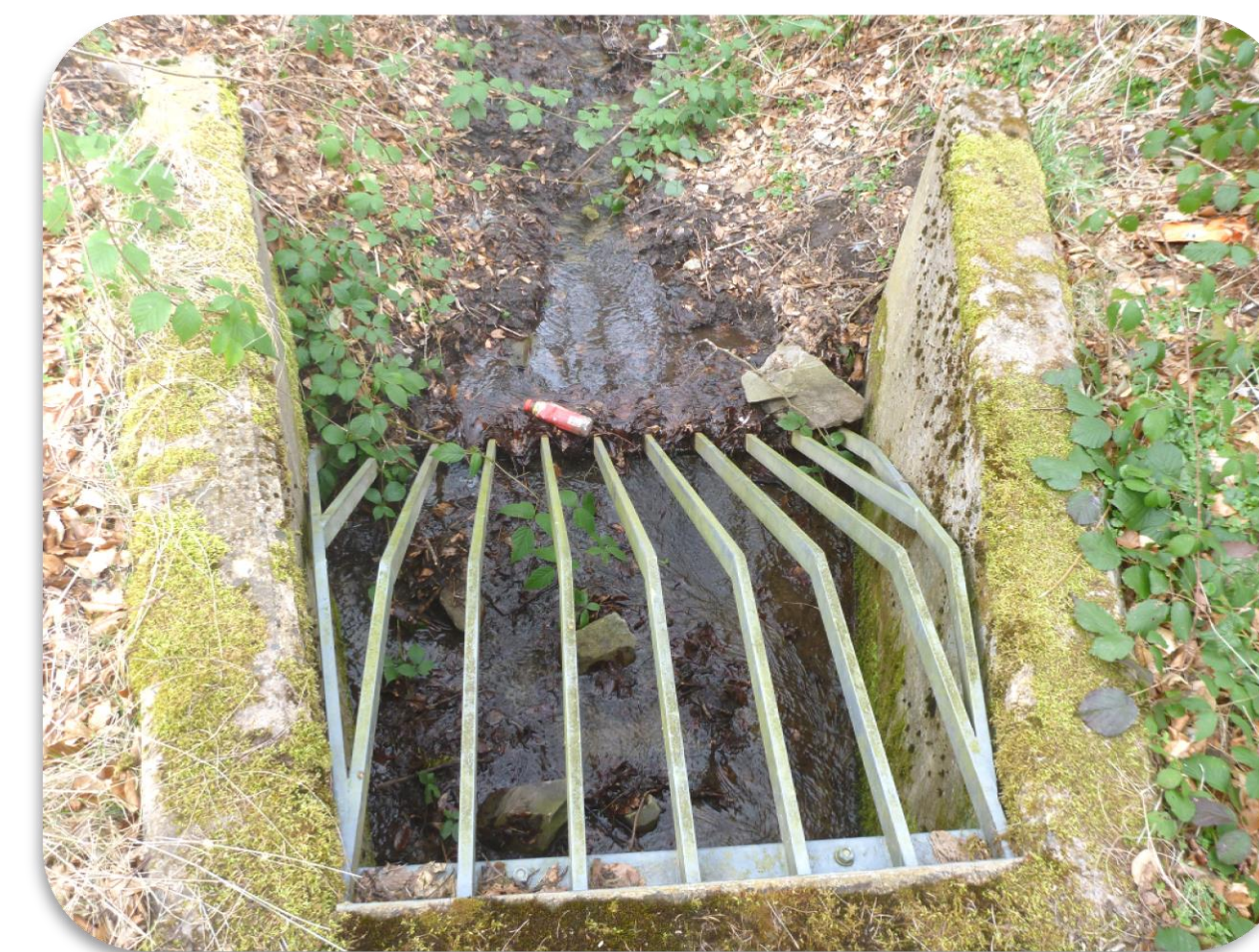
Culverts that constrain flow
