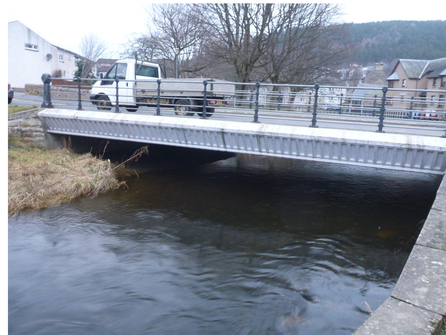
Bridgegate Bridge – little clearance for flood waters below
